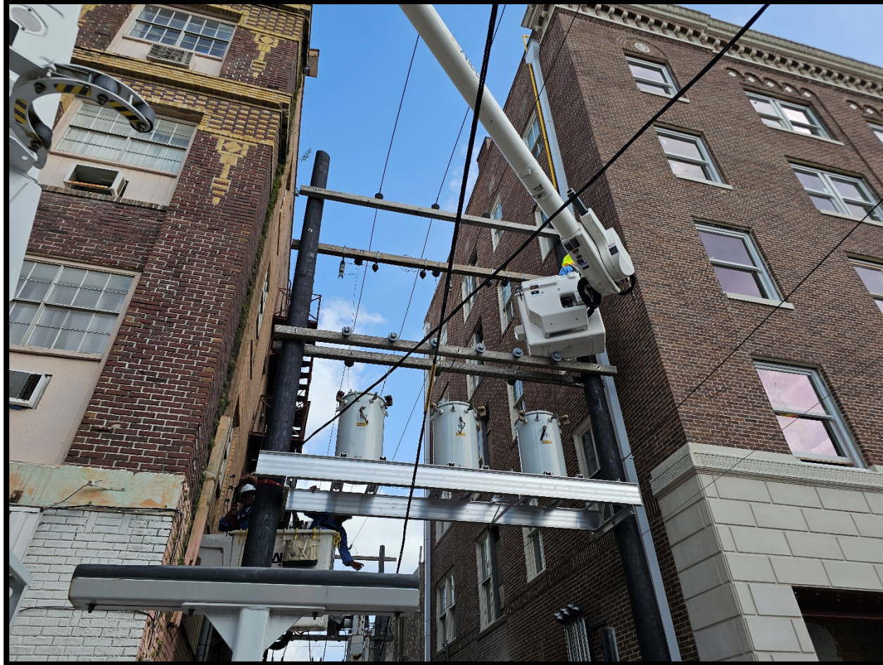
Figure 11. Overhead Transformers Install on H-Frame Structure (Samano Building – Downtown)
