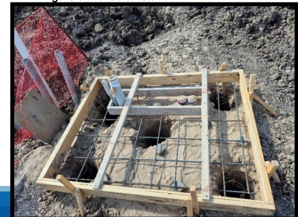
Figure 7. Transformer Concrete Pad Frame
