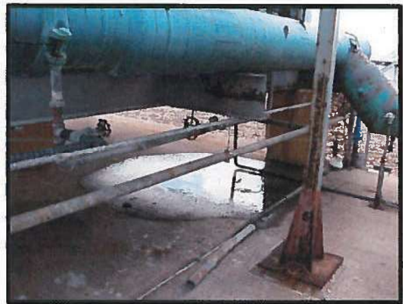
Picture 4 Piping supports showing corrosion and water from basin leaks.
