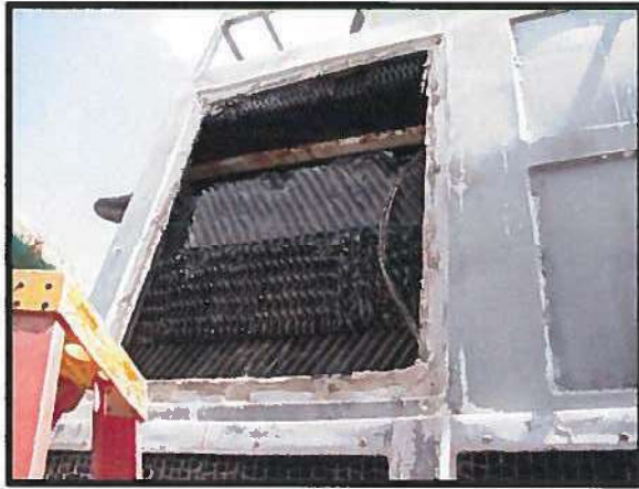
Picture 7 Corroded cross member supports.
