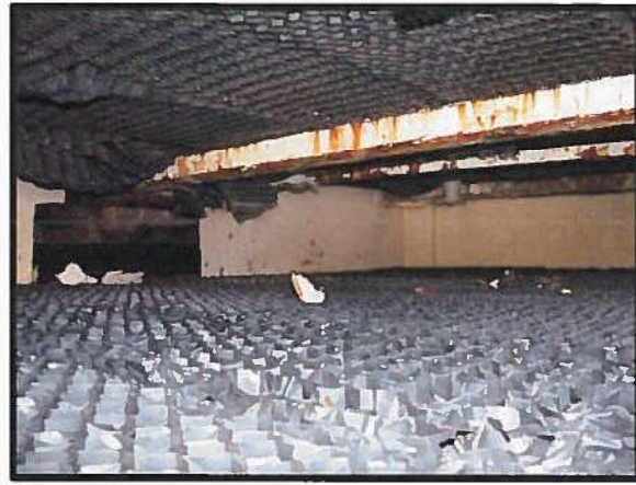
Picture 8 Damaged CT fill and drift eliminators.
