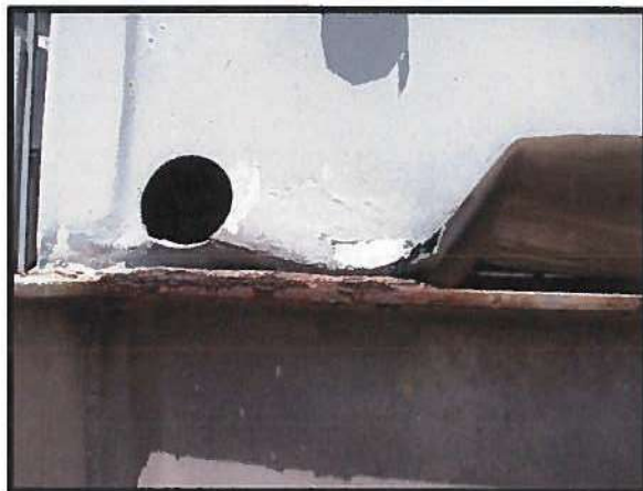
Picture 5 Corner of basin showing cracking of the RFP.
