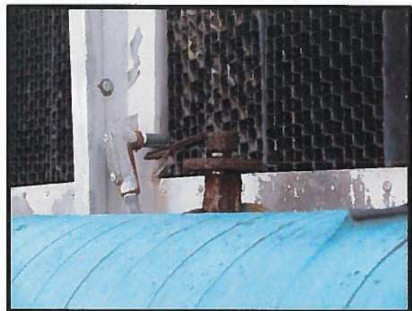
Picture 6 Butterfly valve with severe corrosion rendering the valve inoperable.
