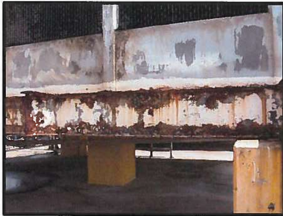
Picture 1 Typical condition of I-beam supports that show corrosion and in some cases thinning of material. The metal has begun to separate in layers of corrosion.
